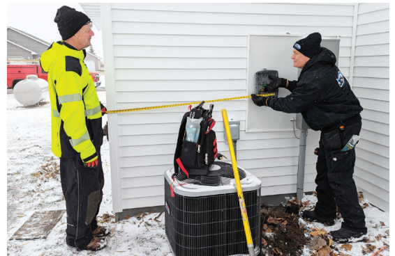
Curt Hyatt and Tom Bolte connect fiber-optic service to a new house in Hoffman.
